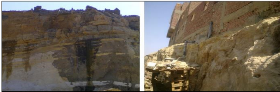
Picture 9: Water Leakage from the Vertical Cliffs in Al-Duwaiqa Area on the Western Slope of the Plateau
