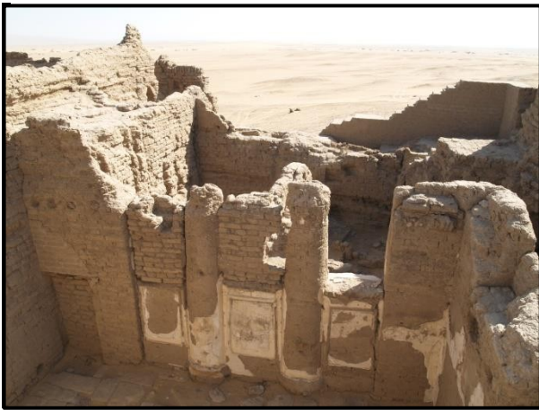
Figure 17. Erosion patterns affecting the upper sections of the Byzantine Church at Doush
