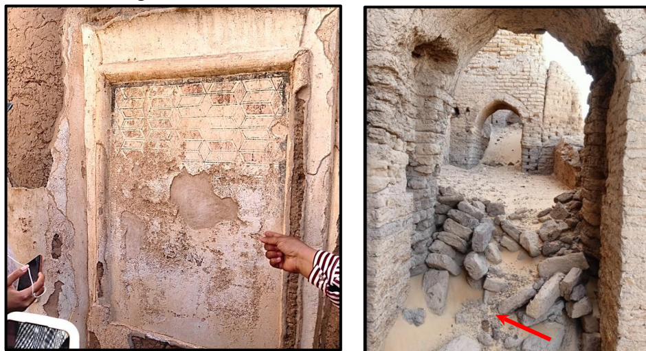
Figure 5. Erosive effects of windborne sand on the Doush Temple structure
